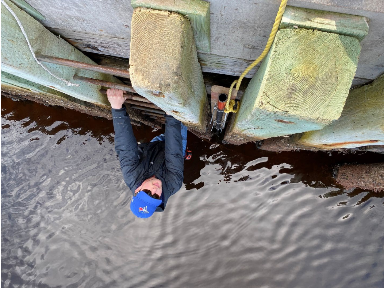
Figure 20 Former AGRG colleague Lucas Mackay on the day of deployment, pictured with the logger deployment structure.
